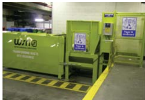
Jones Lang La Salle's Gateway building in Circular Quay is serviced by WSN's Ecolibrium™ business solution.
